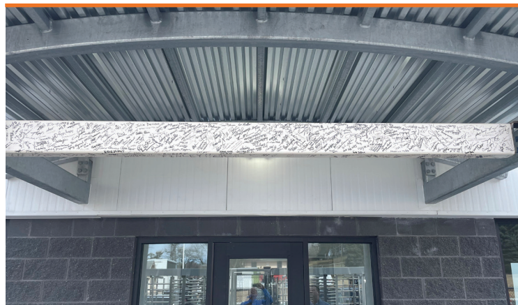
Our recently completed Rochester, MI facility, where employees signed a commemorative beam at the groundbreaking, as seen on cover page, which now hangs at the front entrance to this building.
